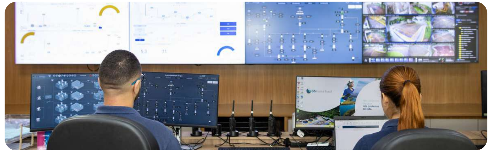
GS Inima Samar Operational Control Center, in Araçatuba (SP).
